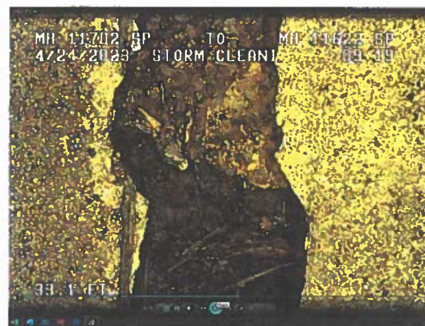
Example of a Failed Segment of Pipe
