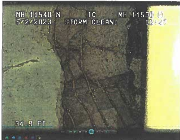
Example of a Failed Concrete Pipe
